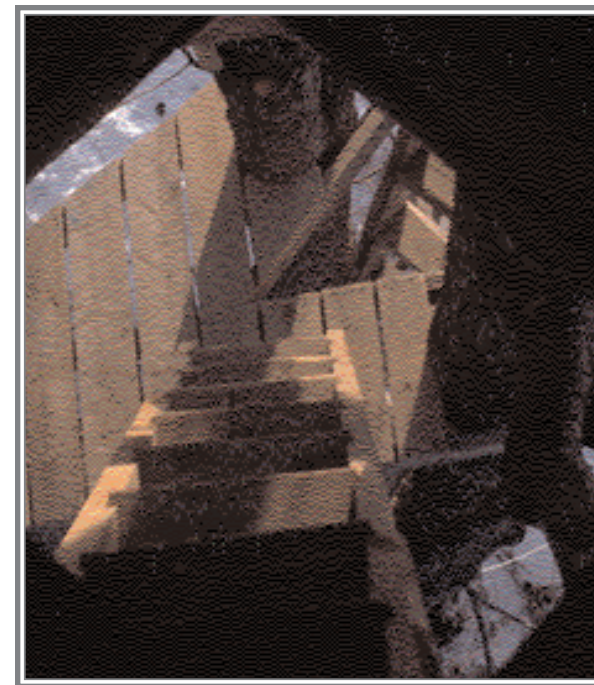
Third ladder run looking down through the trap door in the main floor of the house, towards the second platform.
